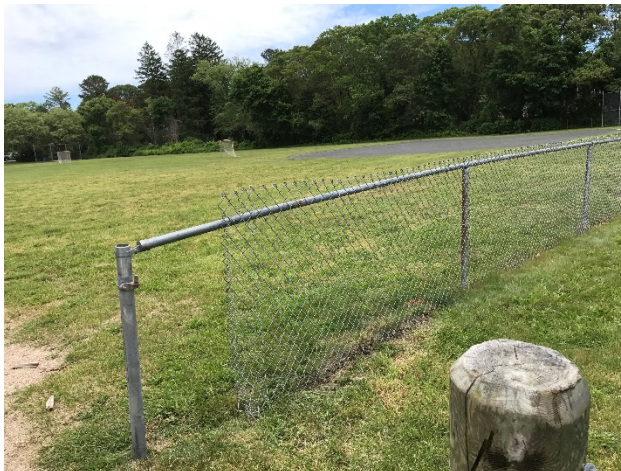
Poor Fencing, Osterville Bay School
